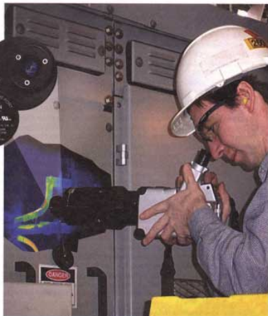
Inspectors at Alcoa's Warrick Power Plant in Indiana can conduct inspections of medium-voltage switchgears through the cabinet door. The infrared camera connects directly to the lens, which presents a wide-field view and provides temperature measurements accurate to ±3°C. It is able to focus on components as close as 2 in. and provides great depth of field, ideal for situations where something is crowded or near the door.
