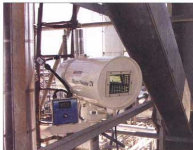
The 14 infrared cameras are located at distances of 10-40 ft from the gas separation unit. They are mounted in totally sealed environmental enclosures with IR transparent windows and continuous purging and cooling by instrument air from a UL-certified air purge system. Real-time radiometric temperature data is transmitted by wireless Ethernet from each camera to a control room 1100 ft away.
